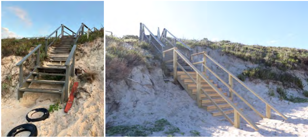
Figure 7-4 Timber Access stairs at Hillier Beach in June 2022 (left) and August 2023 (right)
