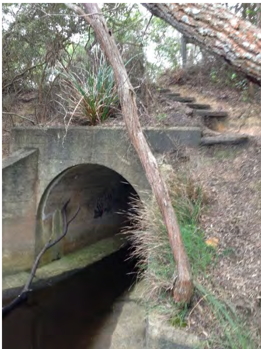
Plate 11 Springdale Tunnel located at eastern end of Springdale Beach Estate Foreshore Reserve
