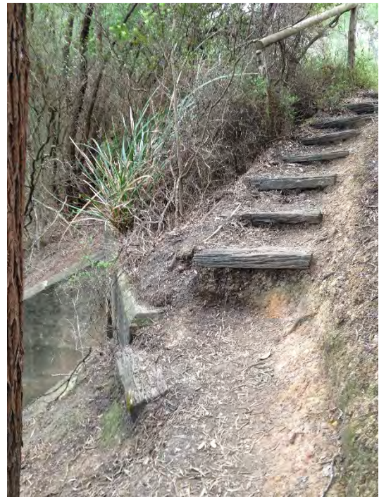
Plate 12 Access to the Springdale Tunnel to the south of the Heritage Trail requires upgrade of steps and handrail
