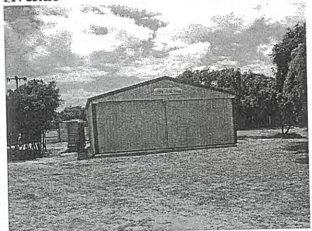
Photo 66 Fire Brigade building on West Avenue This is a large steel building standing alone in a large area of gravel
